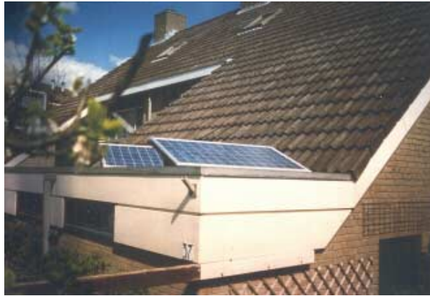
Fig 9. Two AC-modules on the roof of a private residence. A new market for PV.
