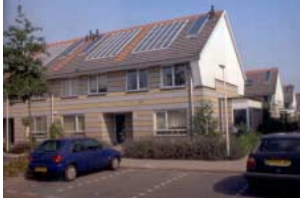
Fig 7. Barendrecht. The first project in the Netherlands featuring building integrated PV on a commercial basis.
