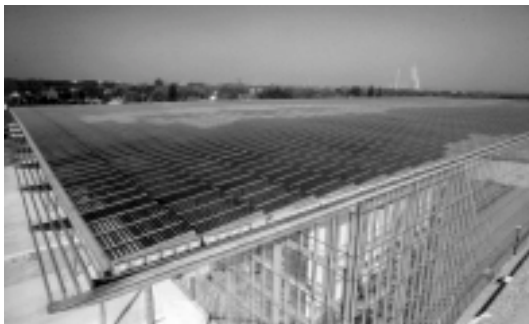
Photo 9: PV-Overhead glazing, 1MWp, Education Centre, Herne Sodingen
