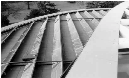
Photo 7: PV-Flat roof integration, 44kW p , Office of the Federal President, Berlin
